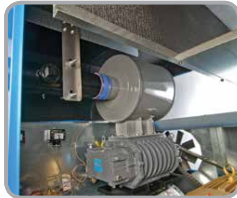
View with rear panels removed
